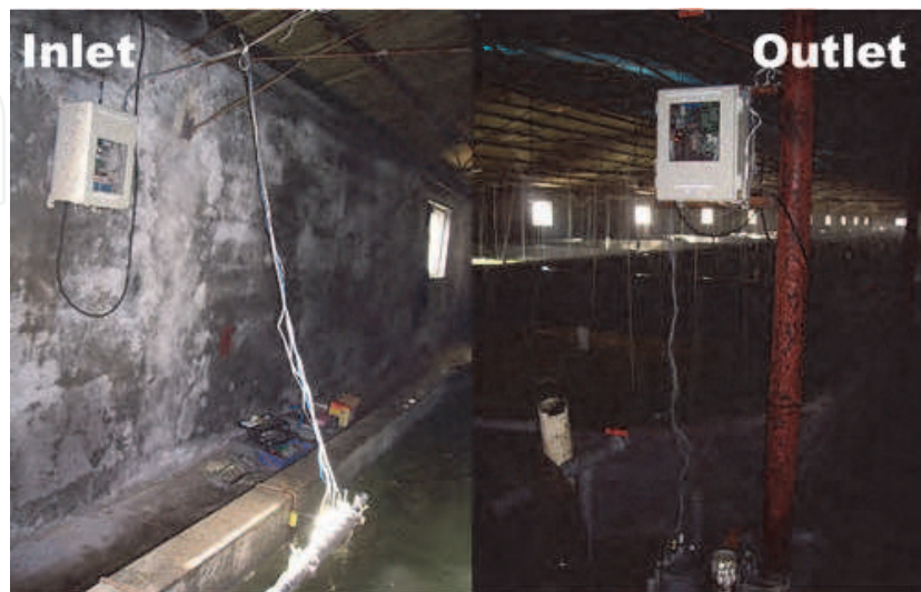
Fig. 7. Water quality dynamic monitoring systems installed in an aquaculture farm.
