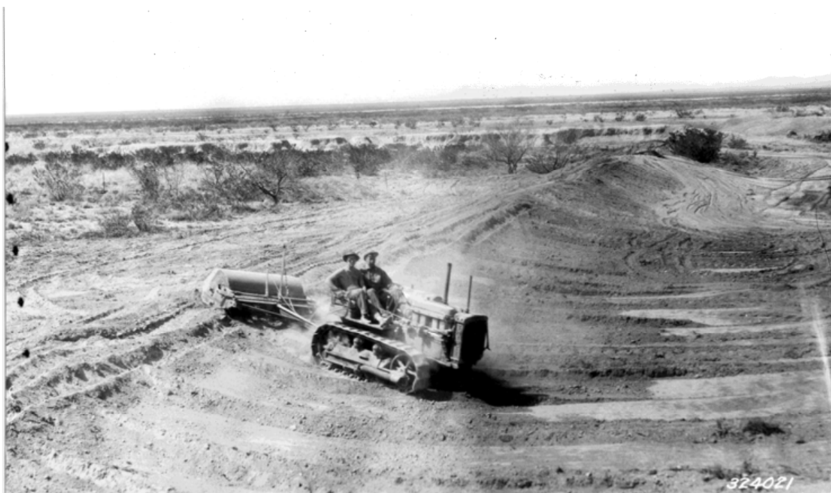
Fig. 5. Use of mechanized earth moving equipment during construction of Big Meadows tank at the Jornada Experimental Range in 1934. New equipment and the availability of the CCC labor force were some of the reasons for the revitalization of water harvesting on rangelands.
