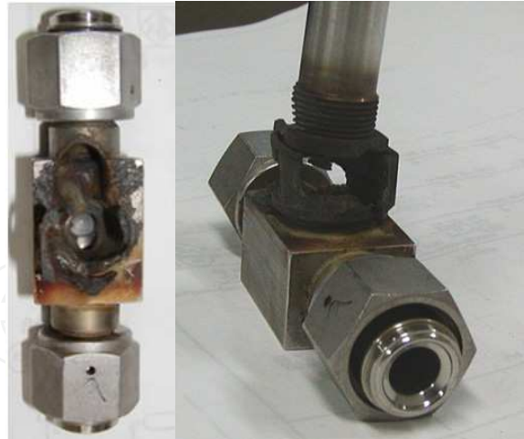
Fig. 5. A burnt valve in a nitrogen trifluoride line caused by adiabatic compression.
