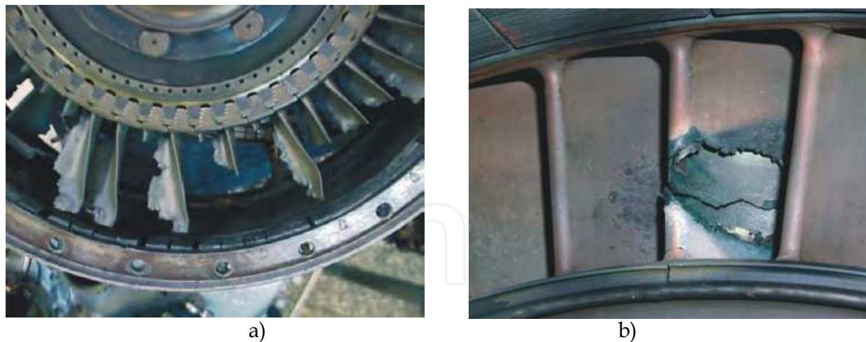
Fig. 8. Characteristic forms of failures to gas turbine caused by long-lasting excessive temperature of exhaust gases (Reports, 2000-2010): a) - burn-through of turbine rotor blades, b) - melting of a nozzle vane
