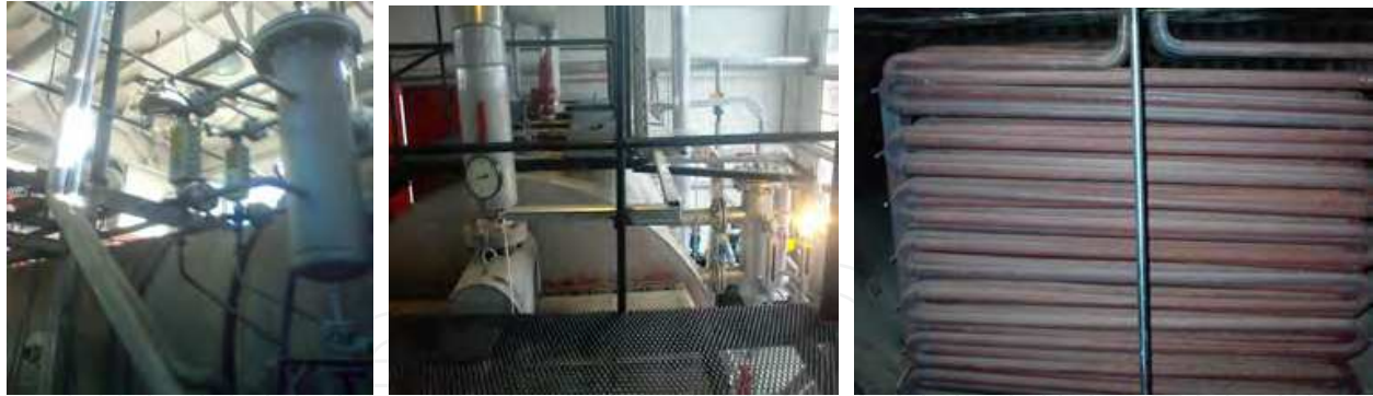
Fig. 3. Superheater of the heat recovery steam generator at 2xST 18 Cogenerative Power Plant
