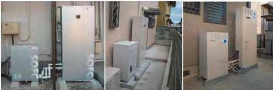
Fig. 7. Appearances of installation sites of residential SOFC CHP systems under demonstrative research project in Japan (Hosoi et al., 2011).
