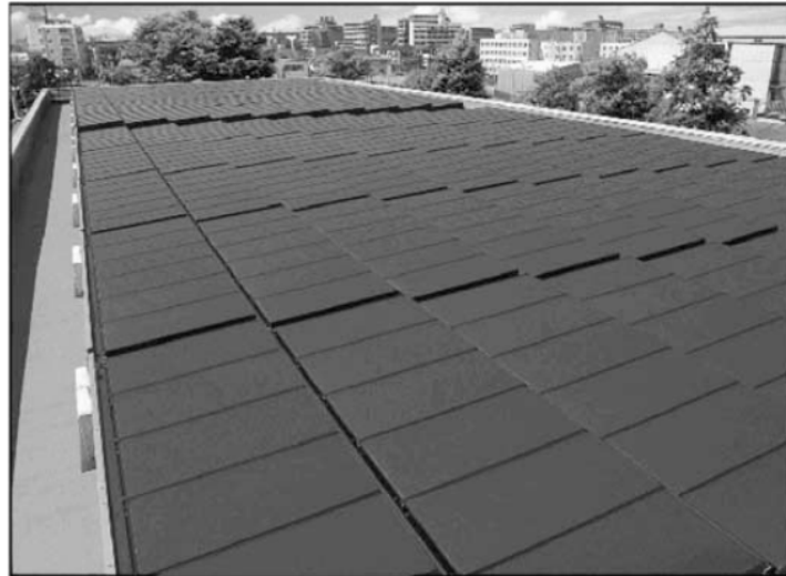
Fig. 10. KW system at the top of the building Osaka (HYBRID modules). Note that modules are installed at low angle (5 degree off from horizontal).
