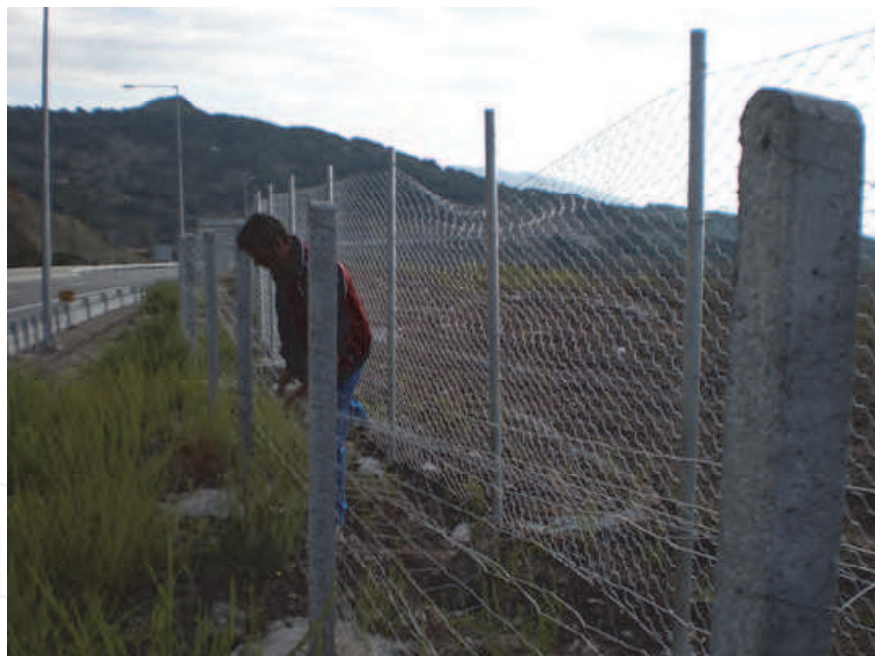
Photo 8. New fence permeability problems due to inadequate standards (missing of the upper bent part)
