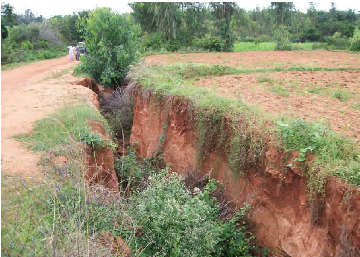
Fig. 10. Neglected road side water drain forming into a huge gully
