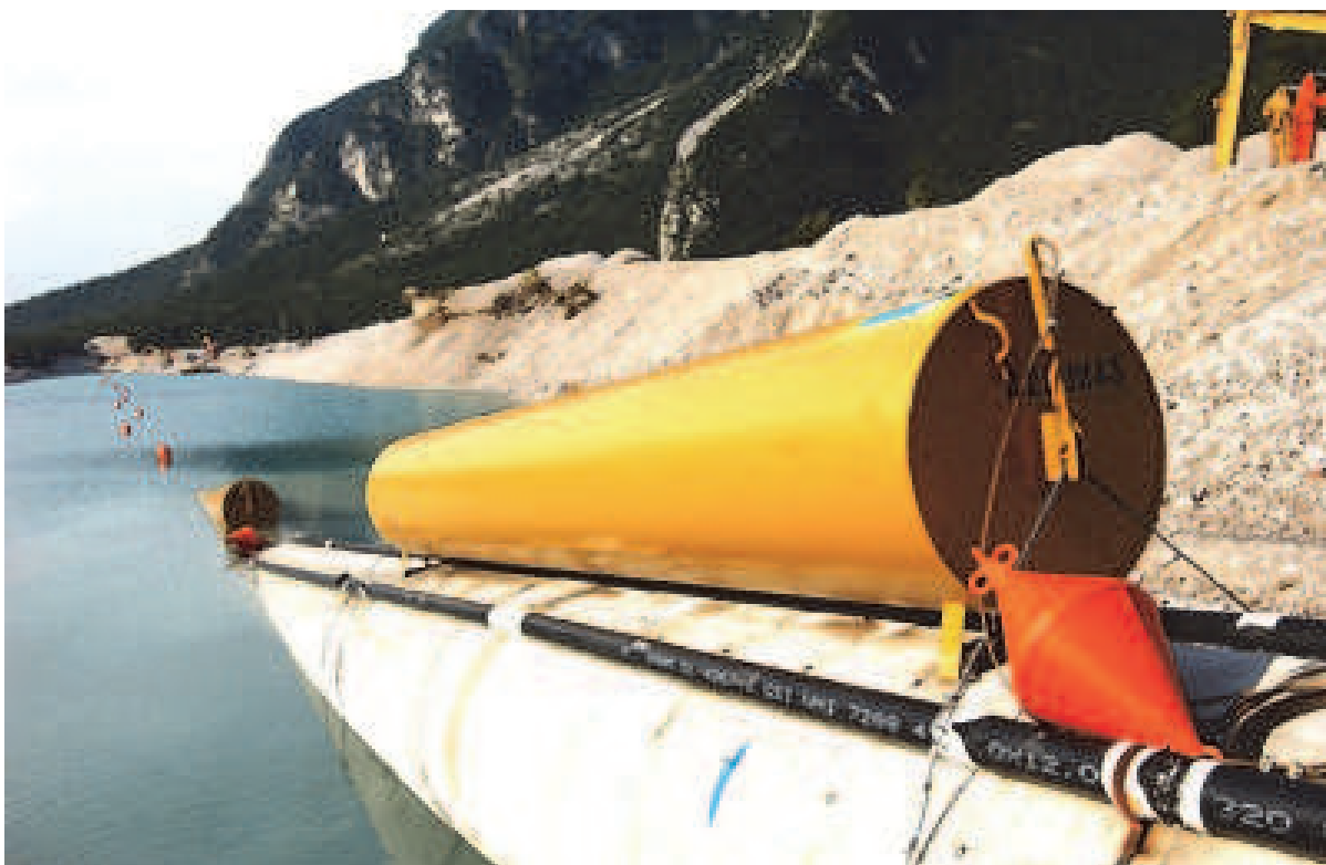
Fig. 2. Launch of a submerged methan pipe. The buoys along the launched lenght are in full view.
