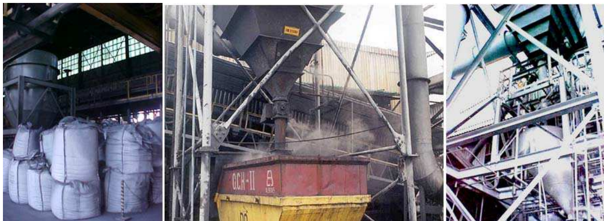
Fig. 15. Petro coke handling problem at Albras, in left bake furnace, in center and in the right bag house dust discharge at the rodding shop - source: Albras Alumínio Brasileiro SA.
