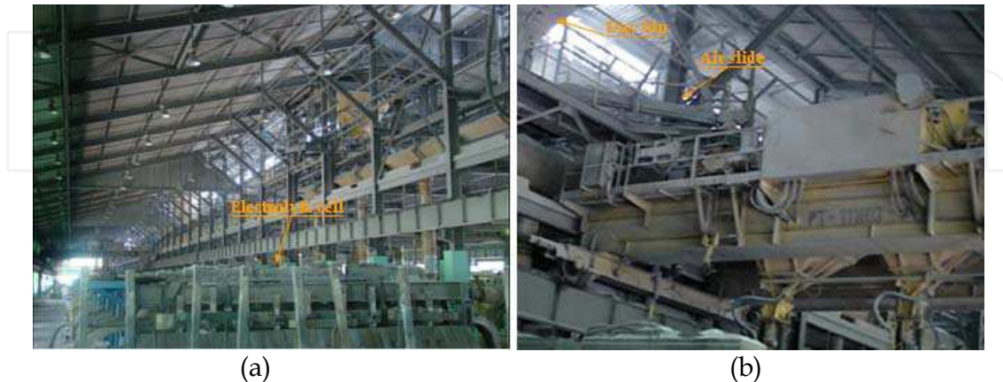
Fig. 2. a) Aluminum smelter pot room, b) Overhead crane being fed of alumina from a day bin by a standard air slide.
