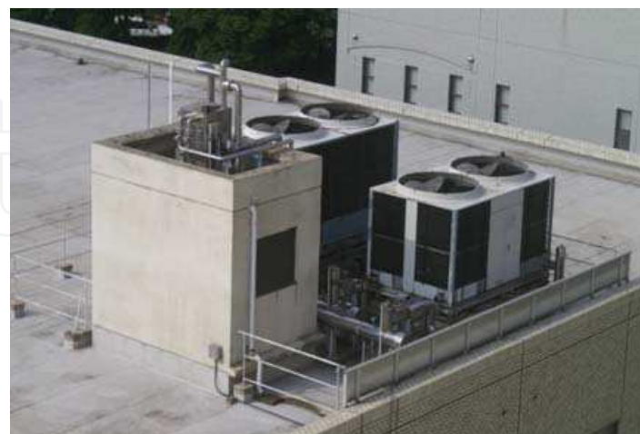
Fig. 14. Heat pump - chiller units
