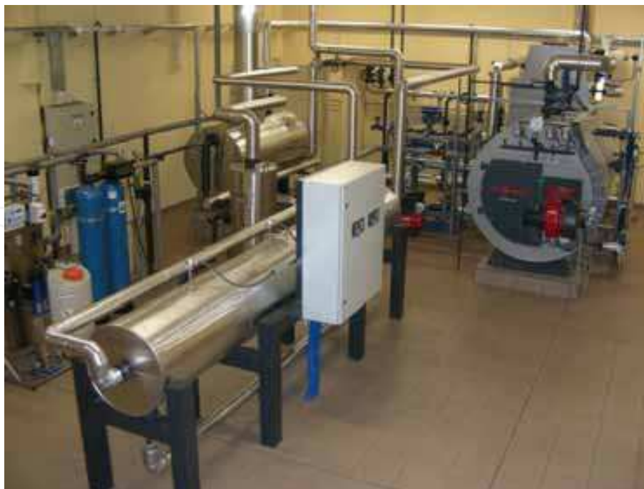
Fig. 11. View of the experimental installation for testing the computer system for on-line monitoring thick-wall pressure components
