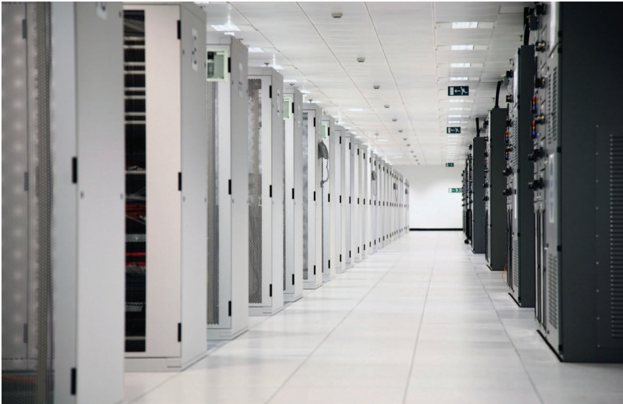
Fig. 1. A large scale data centre with several rows of server racks
