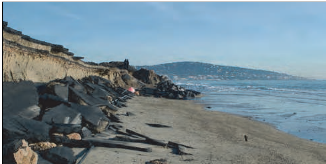
Fig. 12. Frequent destruction of coastal road due to storms (source DREAL LR)
