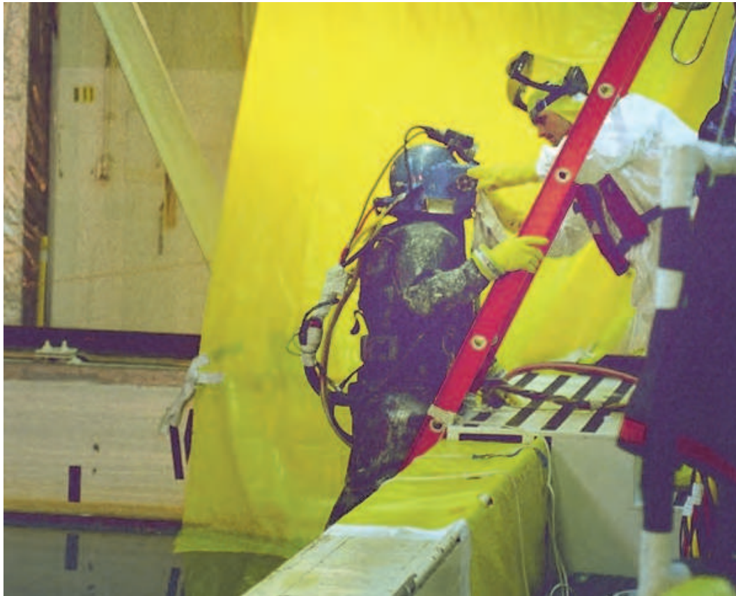
Fig. 1. Diver at INL completing entry into basin for underwater cleaning and coating.
