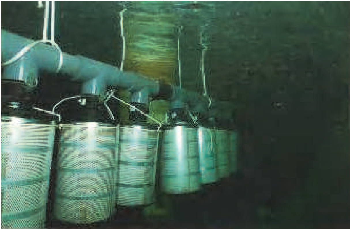
Fig. 4. UCC vacuuming filtration system underwater manifold.
