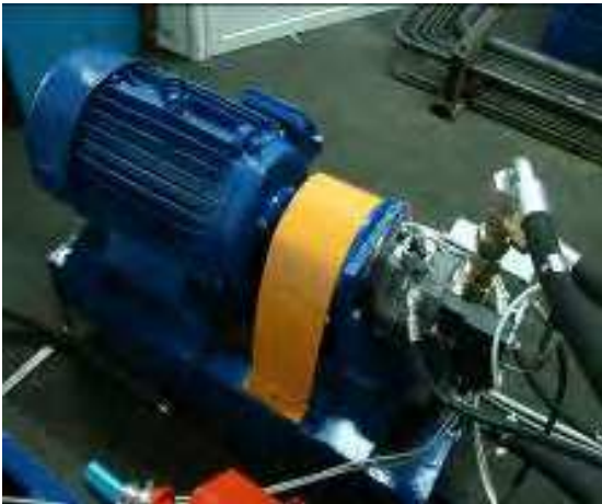
c) Module of the electropump
