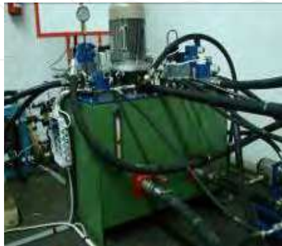
f) The hydraulic station
