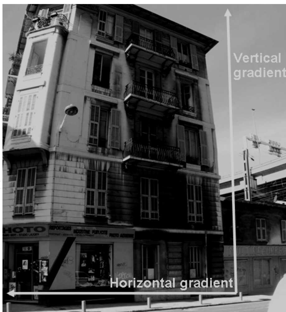
Fig. 3. Building in the centre of Nice, air pollution spatial differentiation (Photo: Gilles MAIGNANT)
