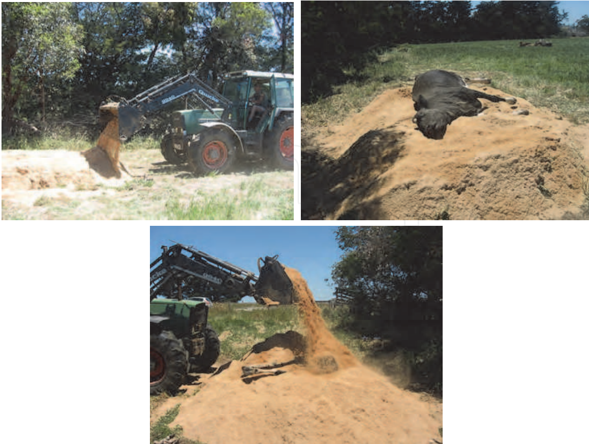
Fig. 6. Construction of compost pile for a large carcass. Photos: J. Biala & K. Wilkinson.
