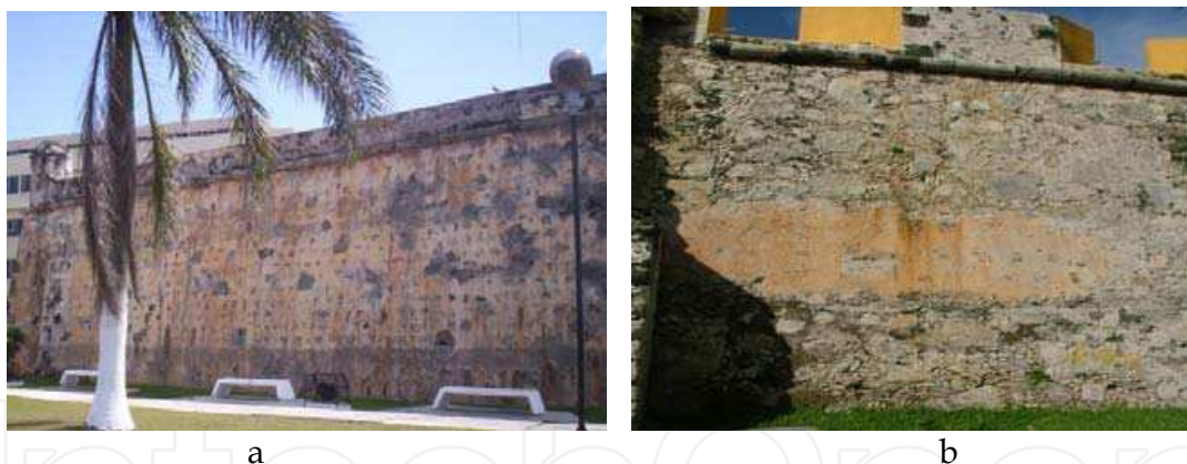
Fig. 2. General aspect of degradation at Forts San Pedro (a) and San Carlos (b), historic buildings of San Francisco de Campeche City.
