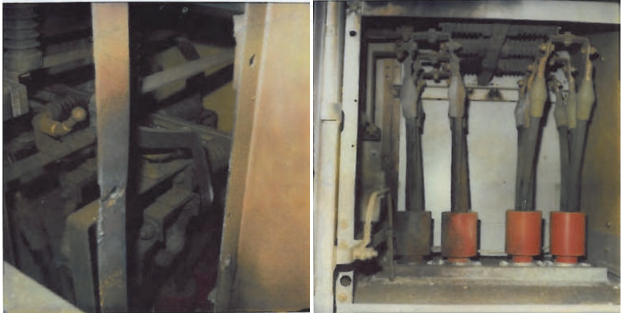
Fig. 5. Photographs: a) view into the exciter cabinet, in the foreground location where the screw loosened and b) view into the cabinet
