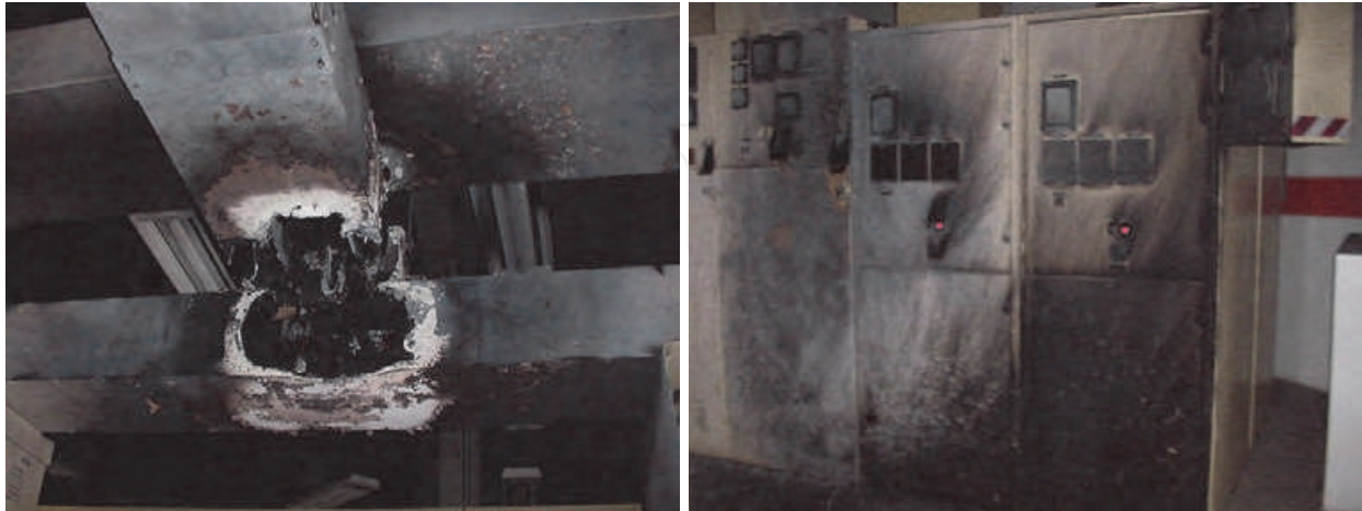
Fig. 9. Photographs of the damages at the Diablo Canyon nuclear power plant (from Brown et al., 2009)
