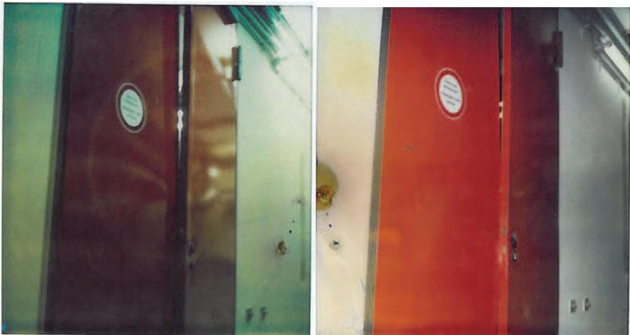
Fig. 6. Photographs of the damaged fire door from outside the room
