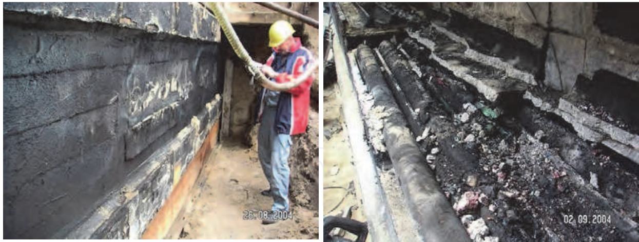
Fig. 3. Photos of the cable damage; left: location of the damaged cable, right: damage by the cable fire/evaporation
