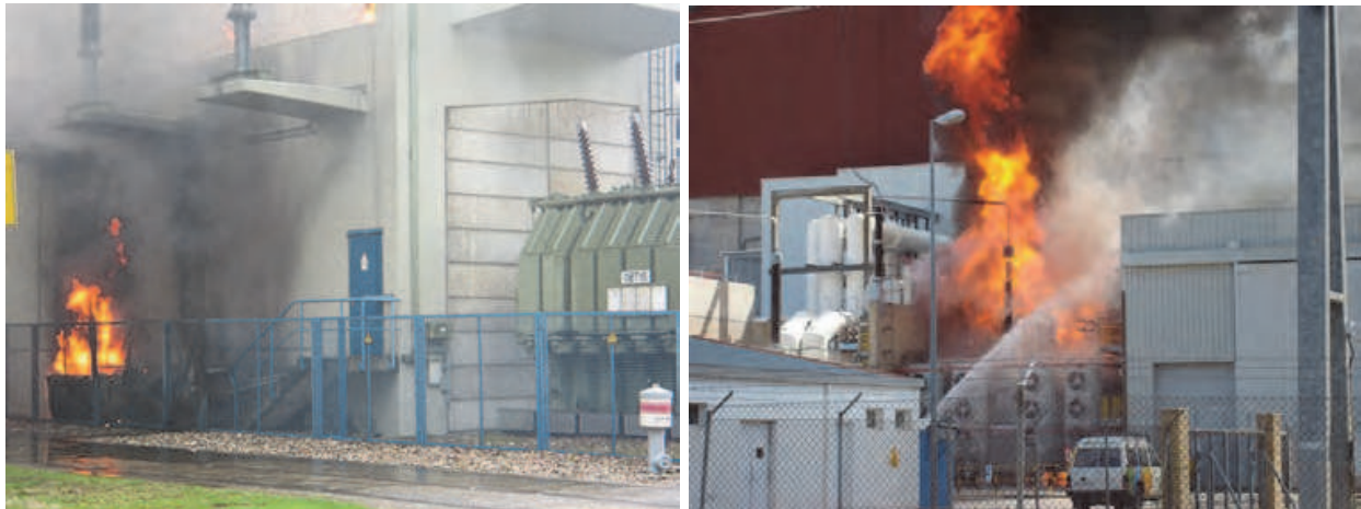
Fig. 8. Flame and smoke occurring at the generator transformer; the photo on the right hand shows the fire extinguishing activities
