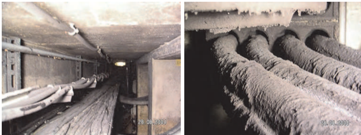
Fig. 4. Cables with protection by intumescent coating; left: photo of the cable channel, right: photo of the coating
