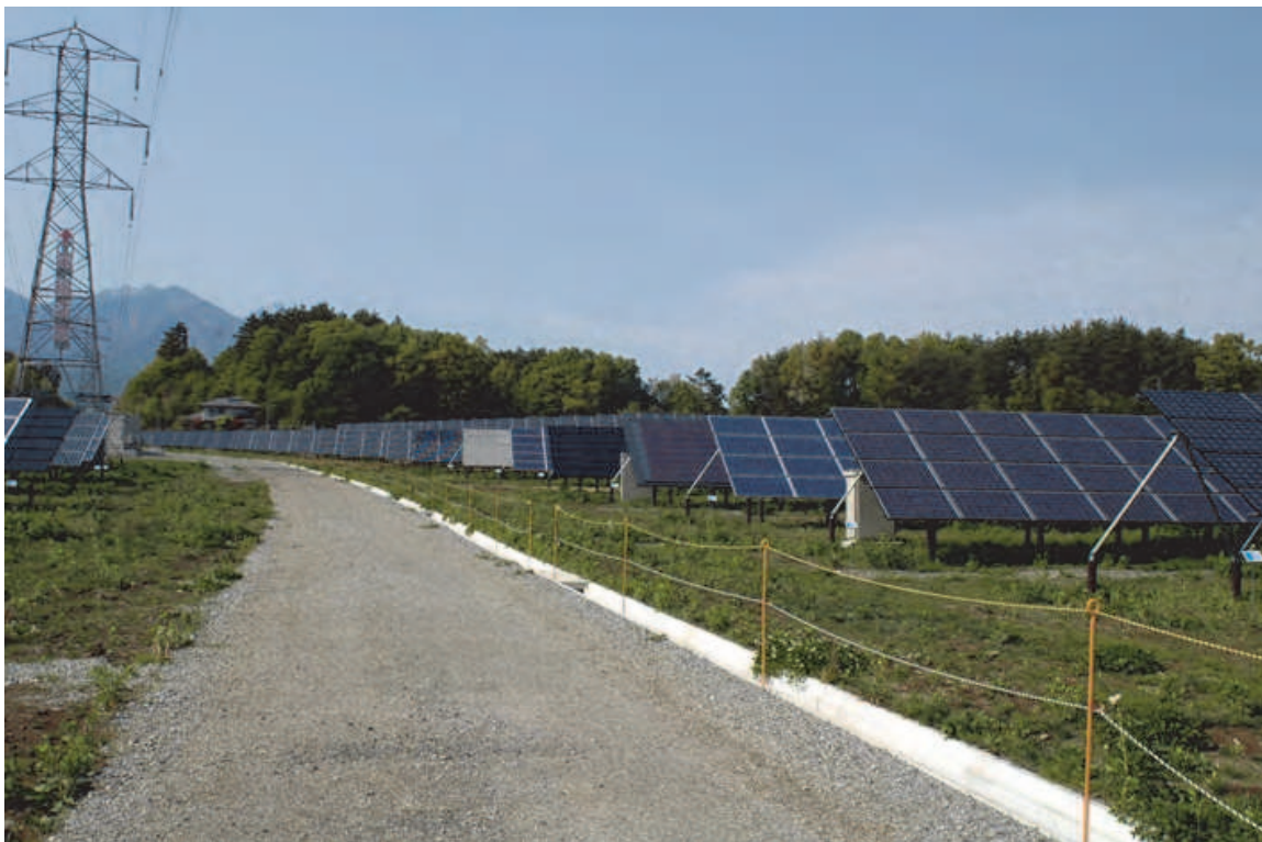
Fig. 4. The 2 MW Hokuto mega-solar plant
