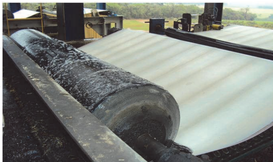
Fig. 5. Blanket type filter system (with suction strainer) to remove water and reduce moisture from the ashes
