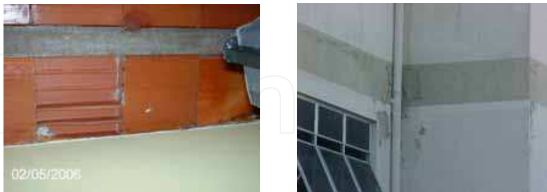
Fig. 3. Detachment of the floor brick and walls
