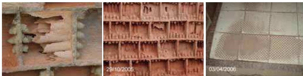
Fig. 4. Fast degradation in masonry due to saline spray and abrasion
