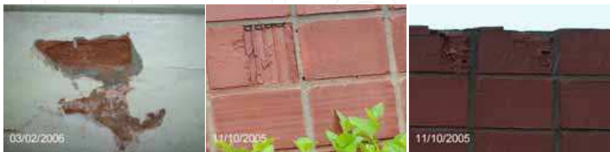
Fig. 2. Fast degradation of masonry due to sulfate water and temperature change
