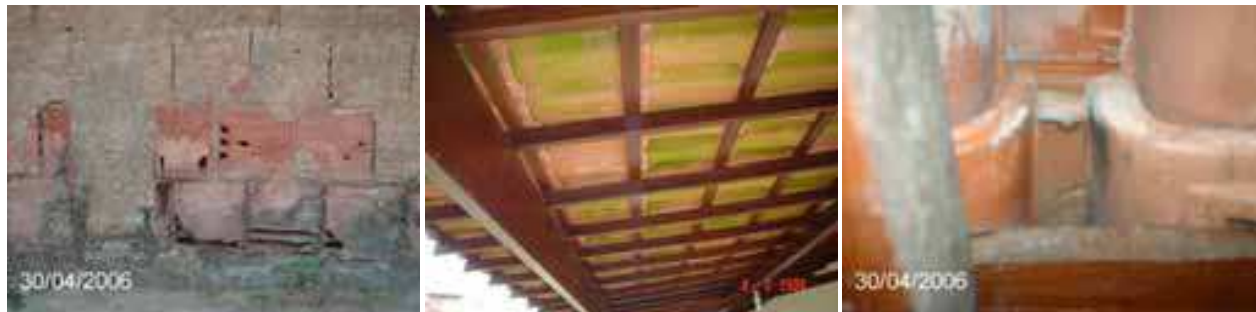
Fig. 1. Fast degradation of masonry and tiles
