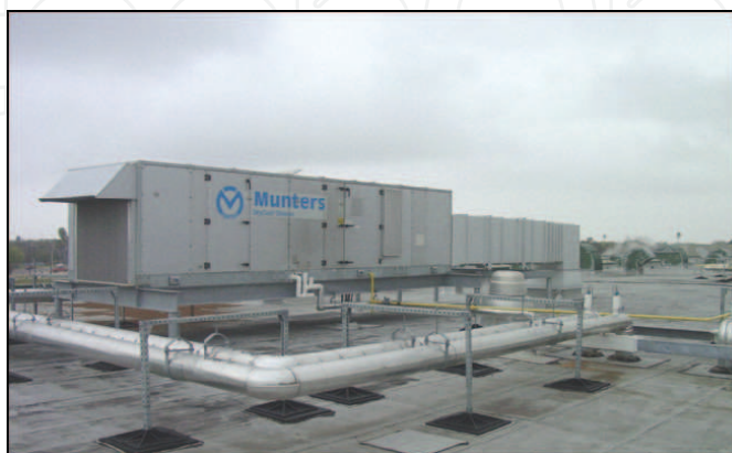
Fig. 1. Desiccant unit installed in a south Texas school to provide pre-conditioned fresh air for ventilation.
