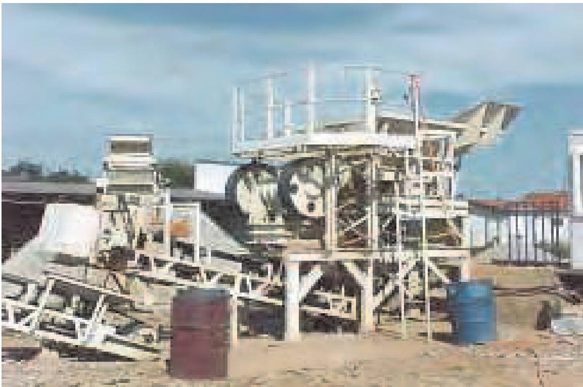
Fig. 7. Plant equipment: a set vibrating feeder jaw crusher + + belt
