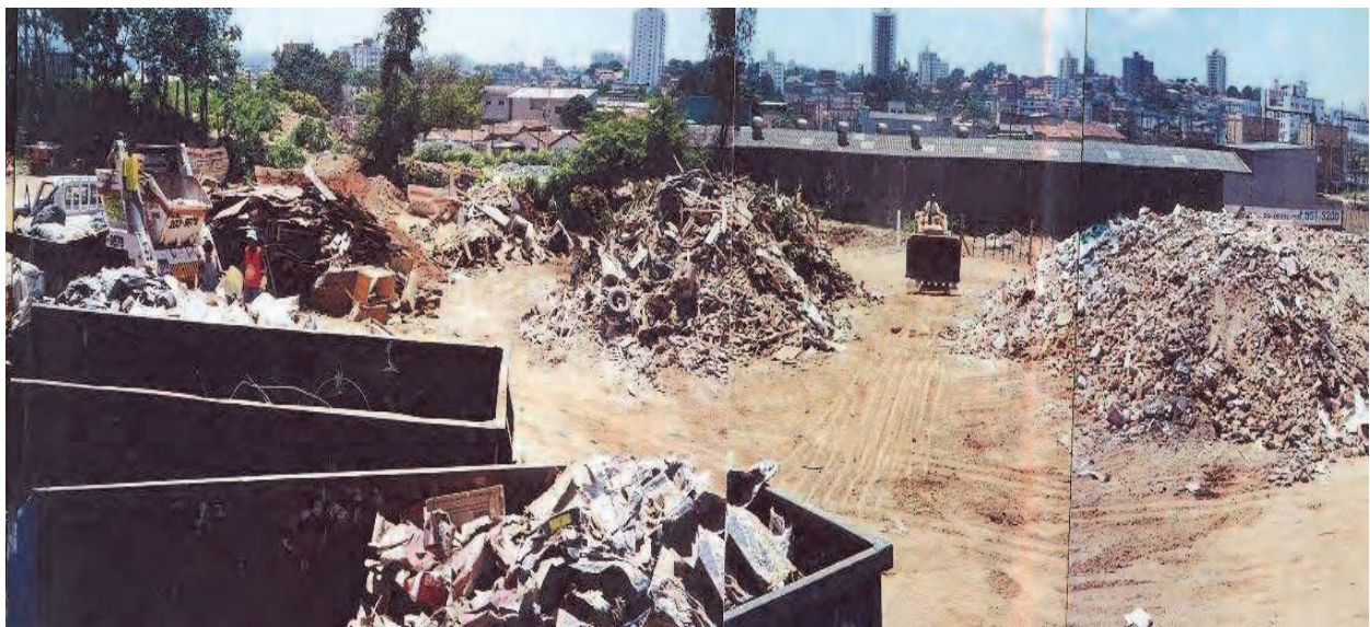
Fig. 5. ATT in the outskirts of Guarulhos in Sao Paulo
