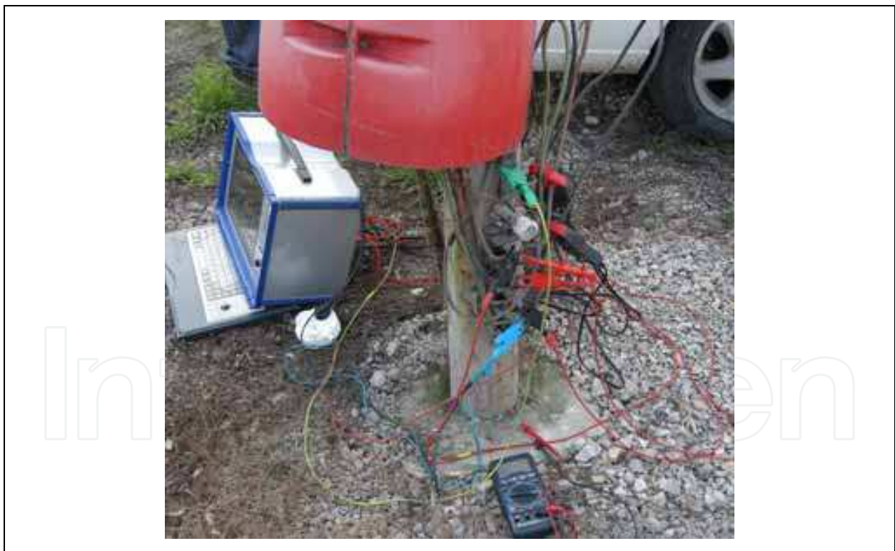
Fig. 15. Measuring power quality in public lighting network
