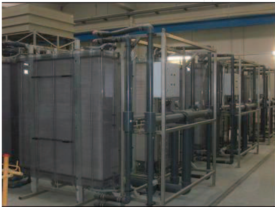
Fig. 4. EDR stacks at the Depurbaix WWTP.
