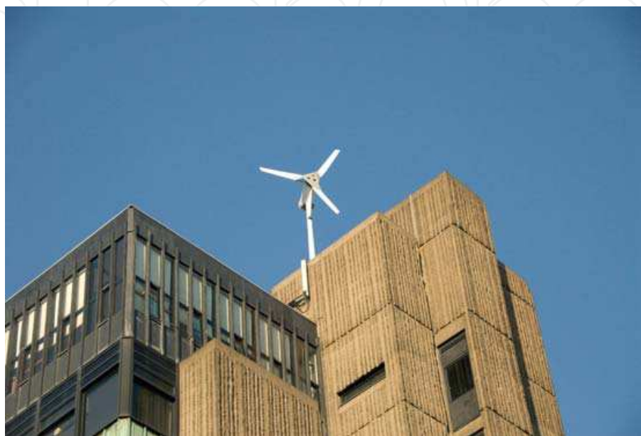
Fig. 6. Roof mounted turbine
