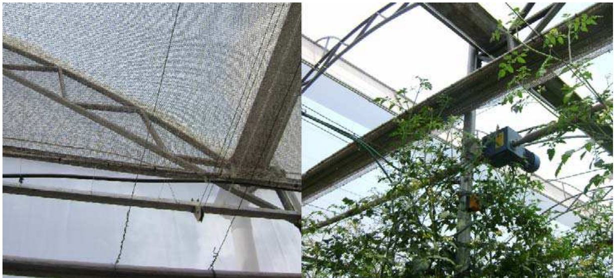
Fig. 8. Elements used for closing and opening the shade curtain including gear motor, pulleys and Raschel net.
