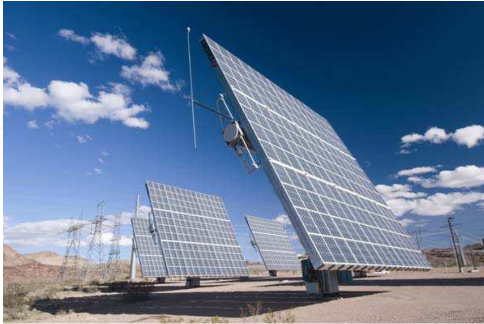
Fig. 16. Installation of CPV systems of Amonix Inc. in Nevada (USA) ( www.amonix.com )
