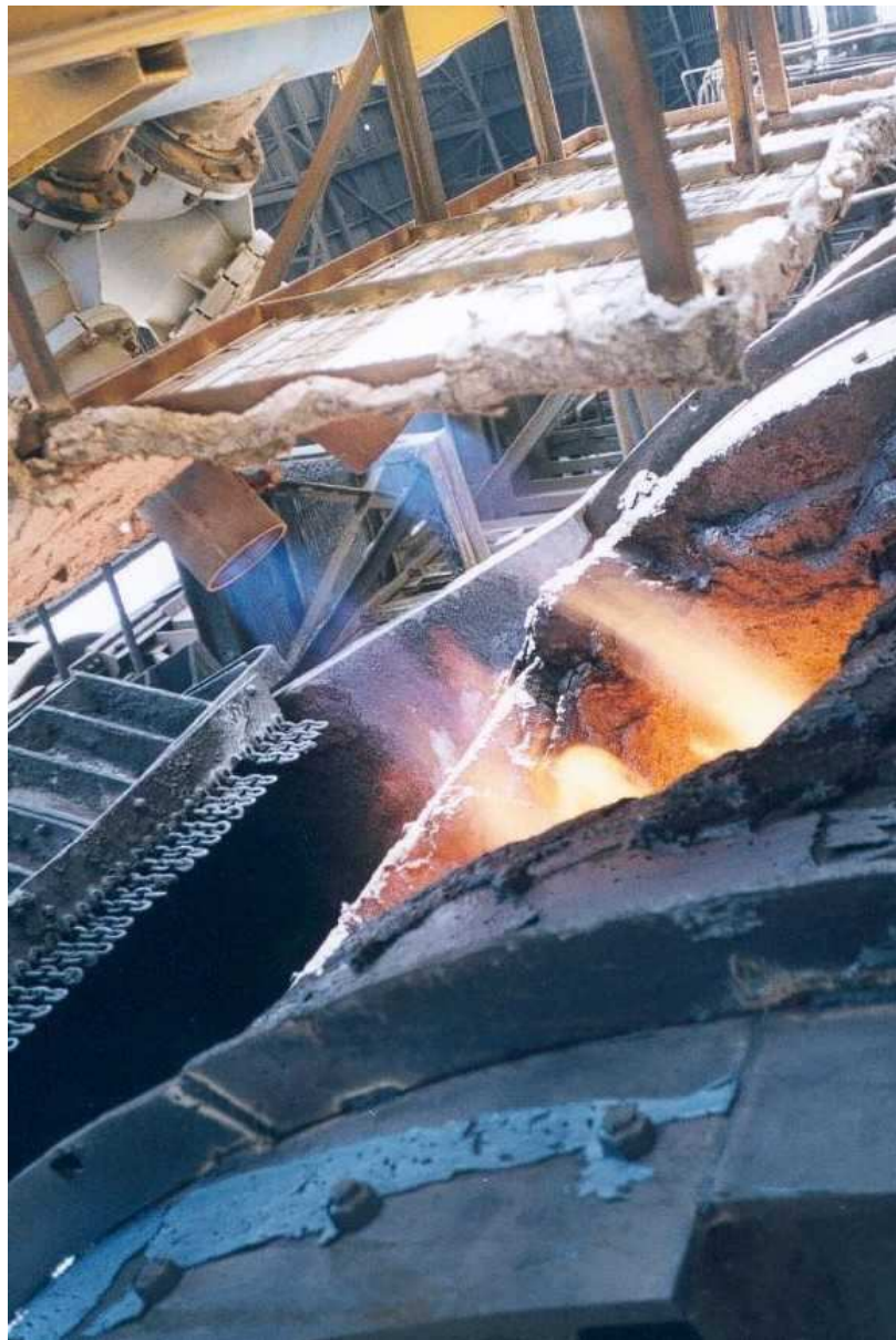
Fig. 7.1 Photo of Burners Installed in P&S Furnace
