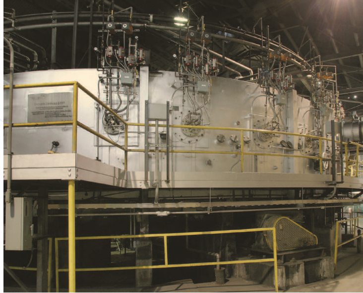
Fig. 10. Outside view of the rotary hearth furnace at ArcelorMittal Shelby after the conversion into all flameless oxyfuel operation. Please note that all bulky equipment and piping relating to the previously used air-fuel system have been removed as it no longer is of any use.
