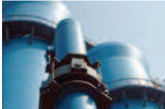
Fig. 6. Blast furnace hot stoves, the large heat exchangers for heating the air-blast to over 1000°C prior to injection into the blast furnace tuyères.
