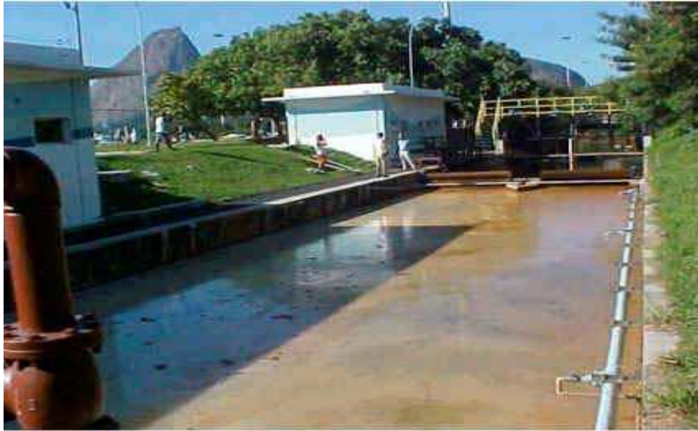
Fig. 4. Treatment station of Flamengo Beach
