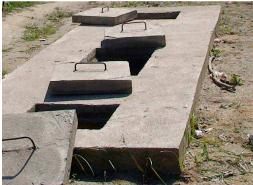
Fig. 7. Photo of the Guerengue road sand filter
