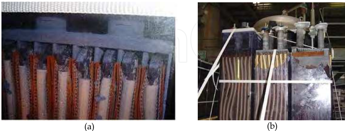
Fig. 5. Due to corrosion, short-circuit took place and caused explosion accident in a standby tubular battery: (a) positive plate lengths were increased and touched the negative collective bar, (b) positive plates were distorted; the positive terminal obviously became more higher than the negative terminal; battery was destroyed after explosion (Source: EDF)
