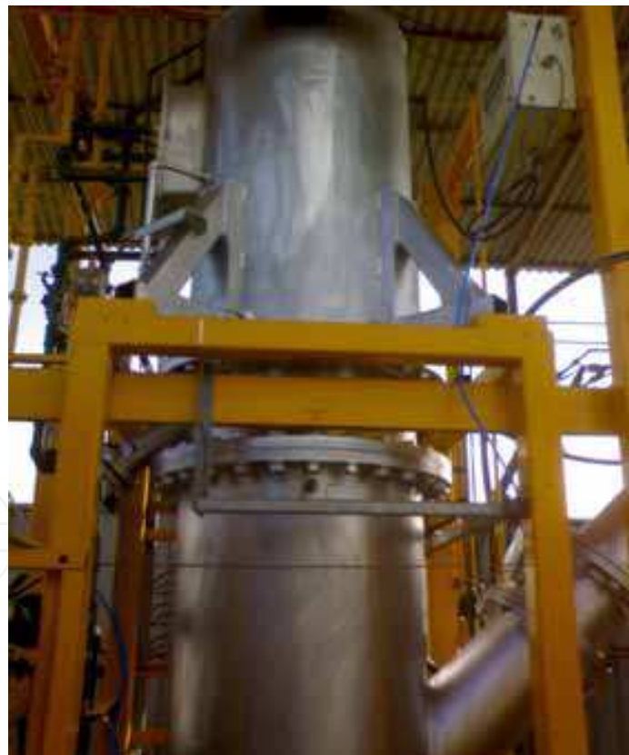
Photo 17. Secondary Combustion Chamber
