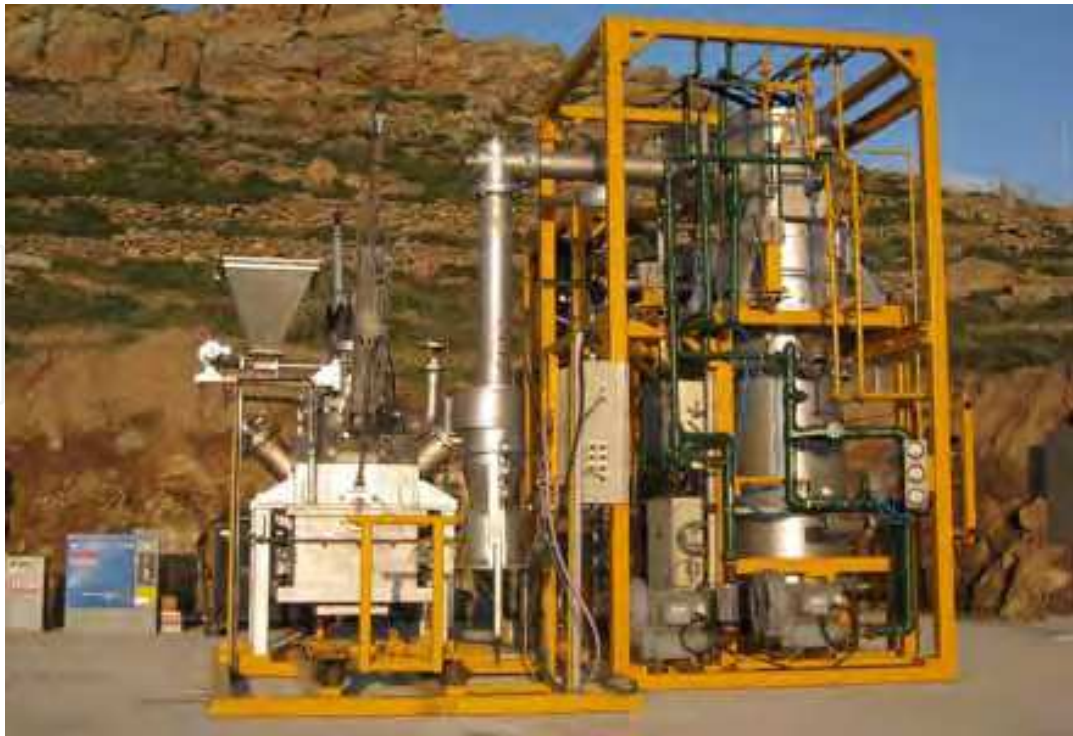
Photo 4. General view of the demonstration gasification / vitrification unit
