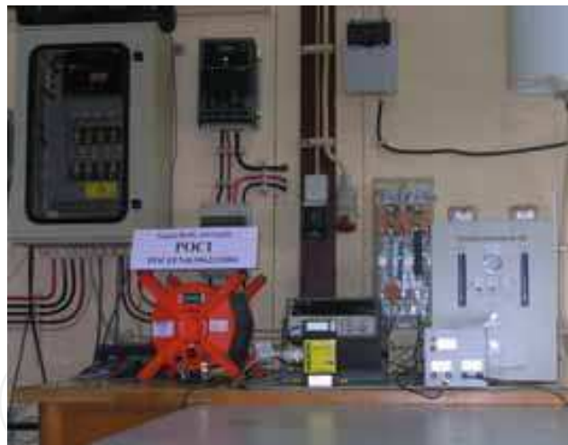
Fig. 4. Stand-alone system's electrolyser, fuel-cell, and electrolyser's DC/DC power converter
