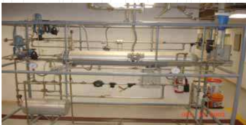
Fig. 17. Industrial heat exchanger used in the experiments.
