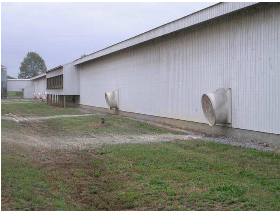
Fig. 6. Fan Arrangement on lower story of hen house. Small extension of building near background has a set of six fans protected to reduce light entry into the building.
