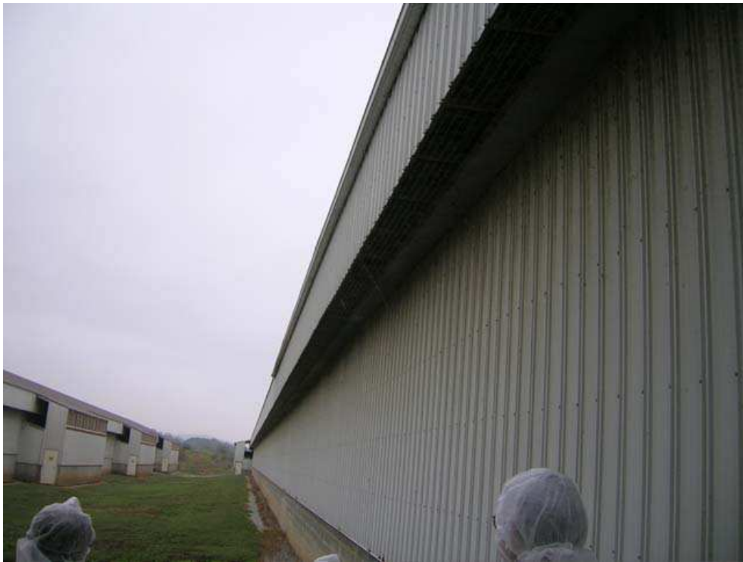
Fig. 7. Open eave along entire length of the poultry house to allow air entry to attic space prior to distribution to building interior.
