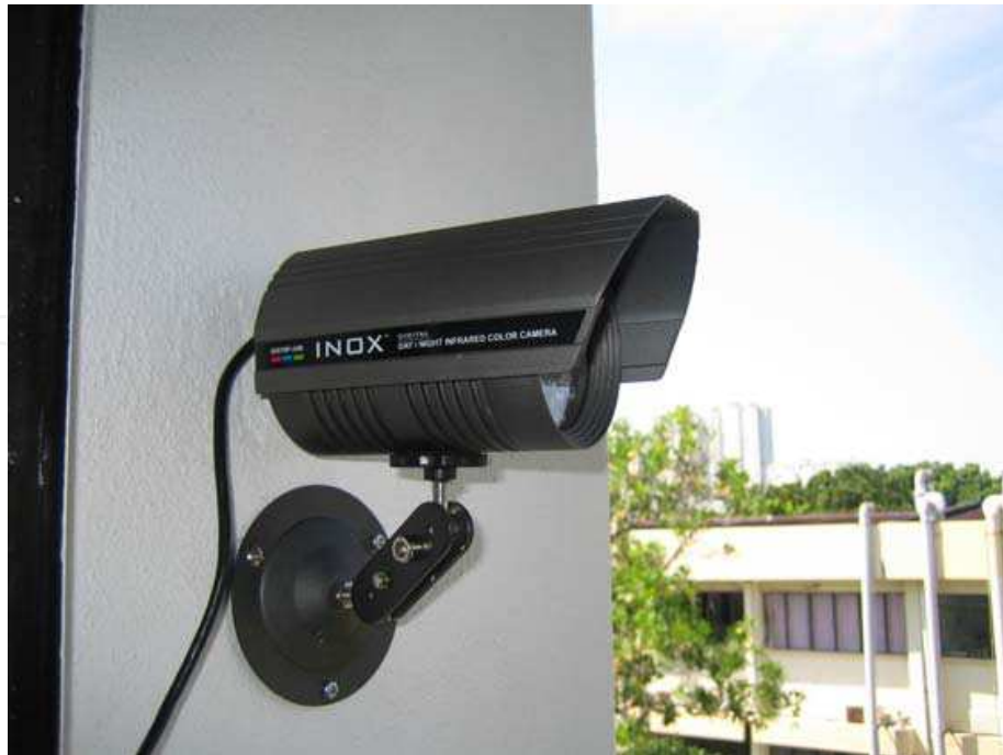
Fig. 2. Internet Video Surveillance (IVS) camera used in this study was installed at the top floor of School of Physics in Universiti Sains Malaysia.
