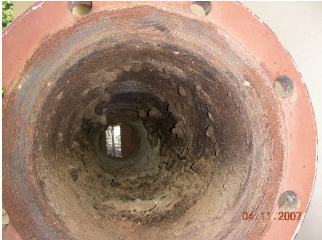
Figure 2. Photography showing the fouling layer formed in a duct section that transports crude oil (Petrobras-BR)
