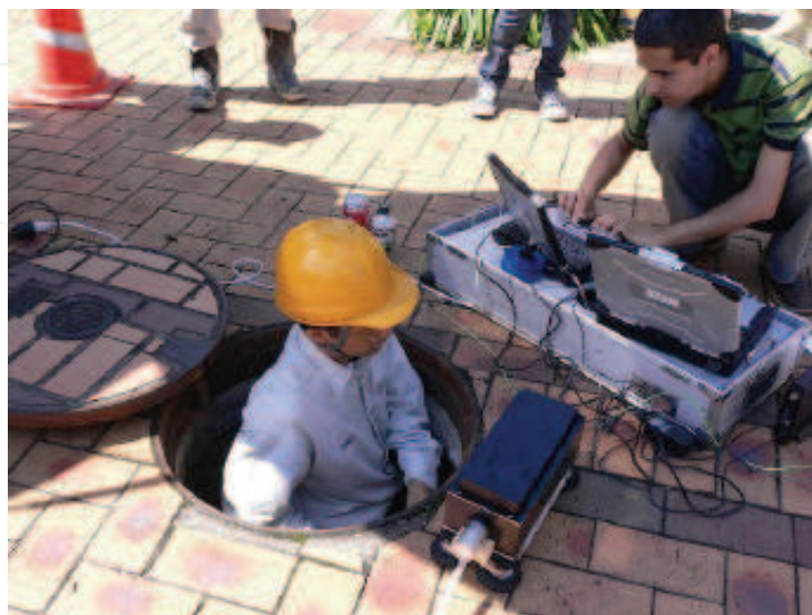
Fig. 17. Scenery of inspection in real sewer pipe net by proposed system
