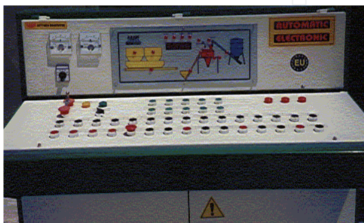
Fig. 12. The central board of plant control and monitoring
