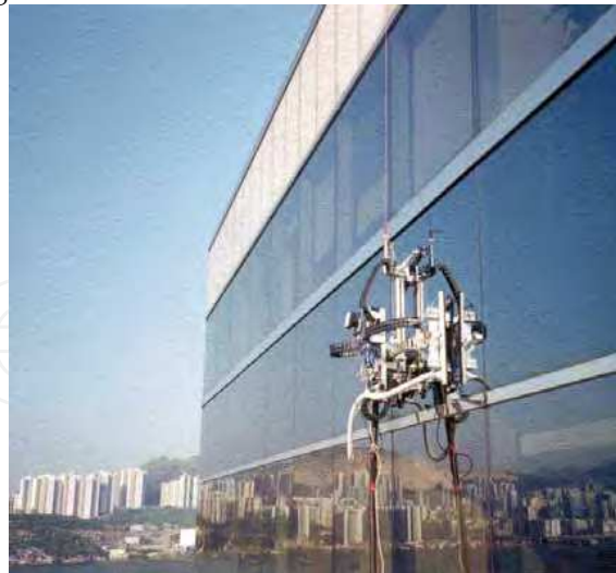
Fig. 3. The climbing robot on site trial outside a commercial building (provided by BBC)
