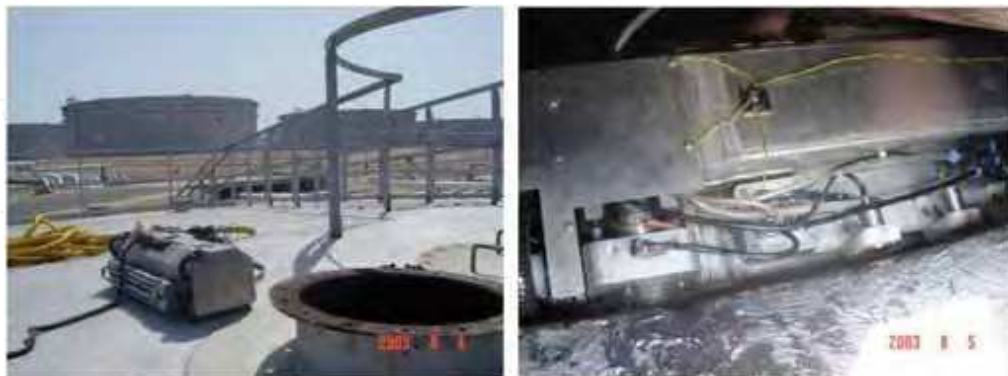
Fig. 6. Left: RobTank before entry through manhole in the roof of a ATG storage tank, Sines oil refinery, Portugal; Right: Ultrasonic NDT tests in oil sludge
