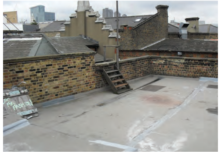
Looking at one of the three platforms
