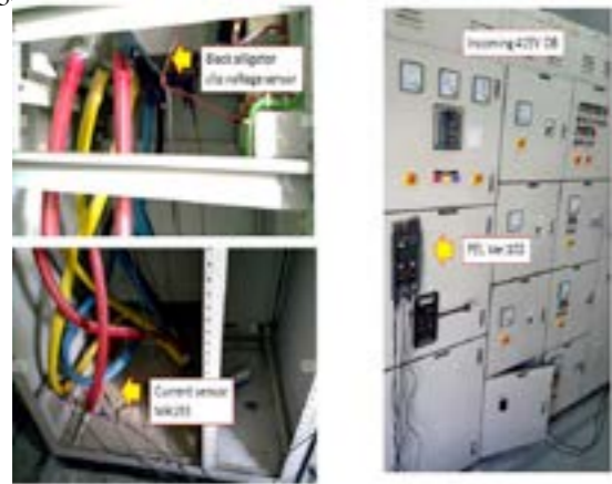
Figure 5: The location of PEL instrument and sensors at the 3 phase electrical room.
