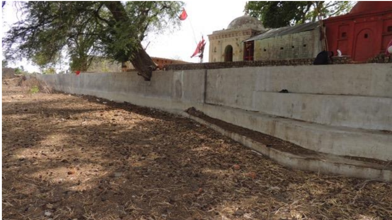
Photo 2: The Haveli, the traditional water harvesting structure is located next to a Hindu temple – therefore Ahirwar (SC) could not attend watershed committee meetings
