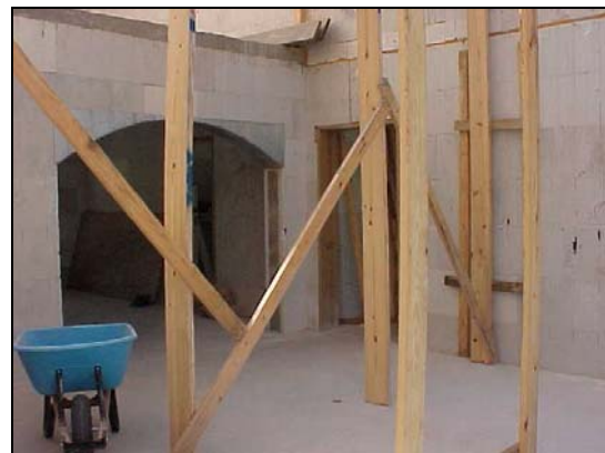
Figure 4.1. Preformed Aluminum Archway in Background; Braces for Wall Blowouts in Foreground
