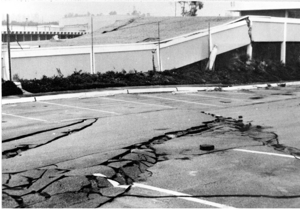
Figure 2.11: San Fernando, California, Earthquake February 1971. Building at San Fernando Valley Juvenile Hall located astride the margin of a lateral spread that produced 3 feet of horizontal ground displacement (USGS 2013).
