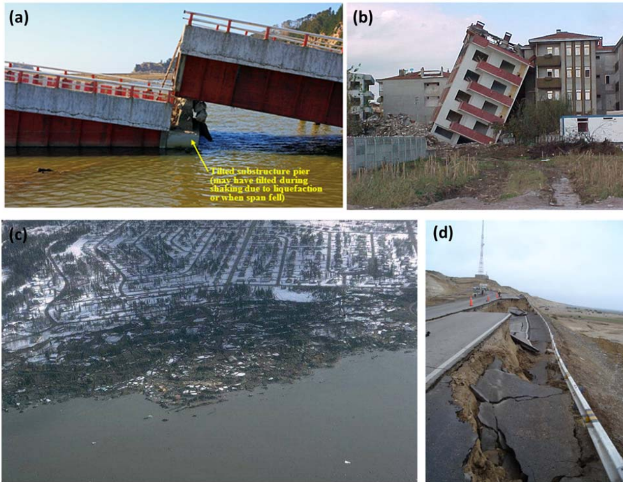
Figure 1.1. Liquefaction damages in built environments. (a) 2014 Chile earthquake ( M_w = 8.8 ). Collapsed and shifted spans at Raqui 2 Bridge due to liquefaction. (b) 1999 Kocaeli earthquake ( M_w = 7.4 ). Liquefaction-induced bearing capacity failure. (c) 1964 Alaska earthquake ( M_w = 9.2 ). Liquefaction induced landslide at Prince William. (d) 2007 Peru earthquake ( M_w = 8.0 ). Liquefaction and lateral spreading of the marine terrace induced failure of the Pan American highway embankment fill
